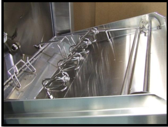
BEDPAN RACK MUST BE IN THE DOWN POSITION
